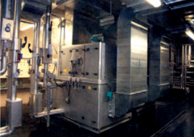
❖ New air treatment unit..
